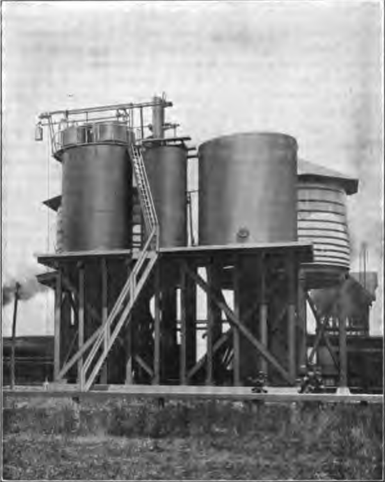
FIG. 47.—Water-softening Plant, Middlepoint, Ohio—Pennsylvania Lines West of Pittsburgh.
